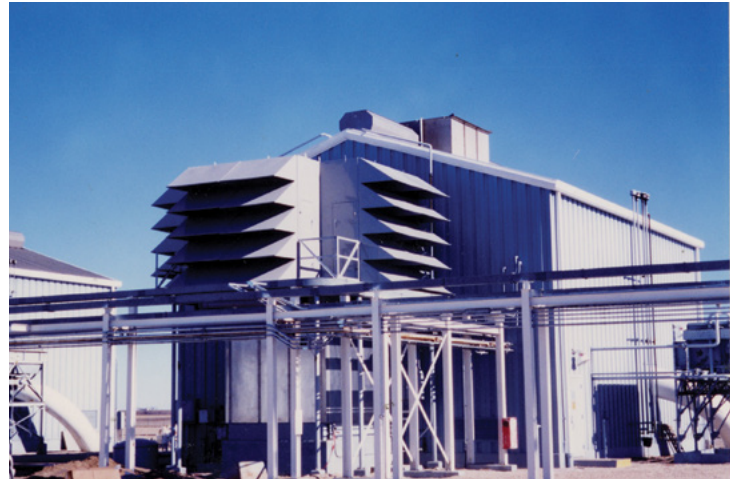
A GTAf 75 retrofit installation for a 13,500 hp Rolls Royce Avon turbine station in Wilson, Kansas.
