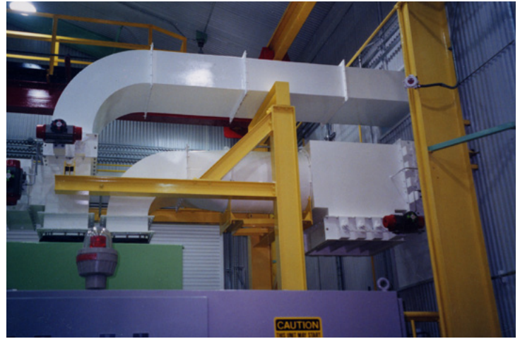
A new construction 1500 Hp, 9600 CFM synchronous motor EMVS installation in Midland, Kentucky. This view of interior components shows the optional diverter unit (large white cube lower right) which redirects discharge heat to warm the compressor station in cold weather.
