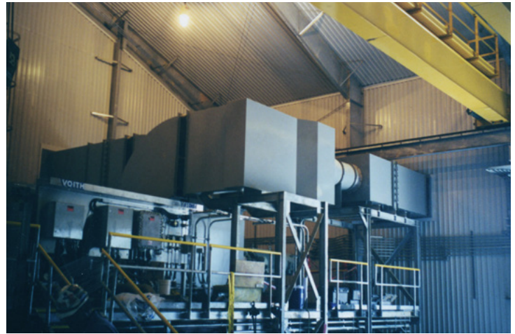
A large, new construction 13,000 Hp, 11,020 CFM synchronous motor EMVS installation for Kinder Morgan in Longview, Texas.
