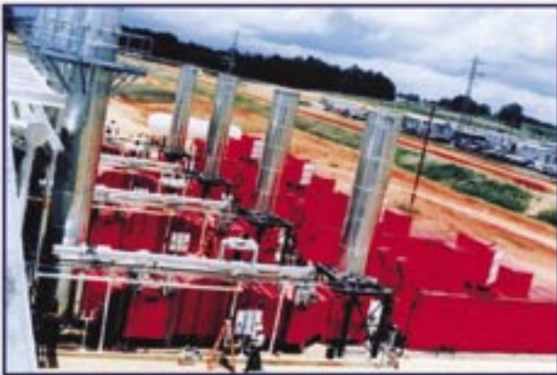
Gas Turbine Skid Enclosure
