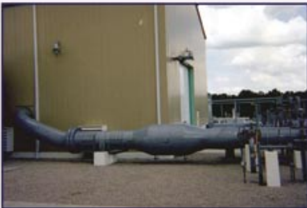
Centrifugal Gas Compressor In Line Discharge Silencer
