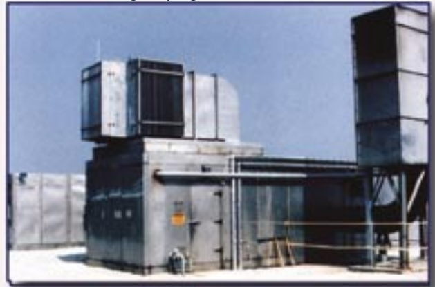
Gas Turbine Intake Silencer
