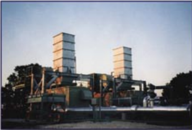
Gas Turbine Exhaust Silencer
