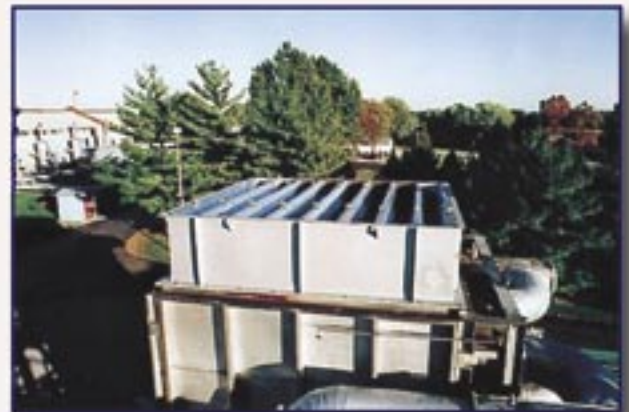
Gas Turbine Exhaust Regenerator Silencer
