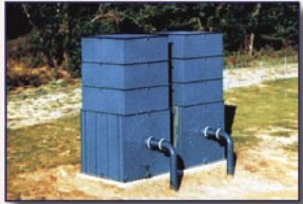
Suction & Discharge Piping and Unit Blowdown Vent Silencer
