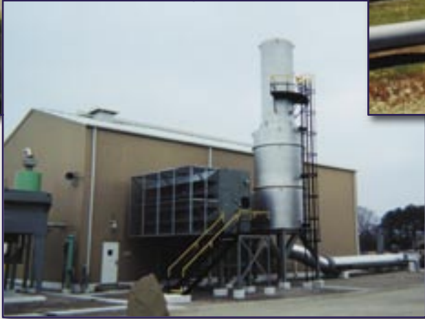
Solar Mars Intake and Exhaust System Designed to Meet 60 dBA at 50 ft. From Compressor Building
