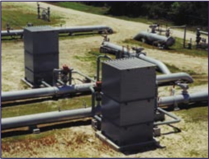
Compressor Station ESD Vent System Designed to Meet 50 dBA at 100 ft.
