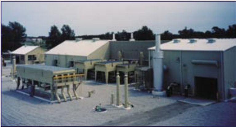
Solar Saturn Intake and Exhaust; Designed to Meet 50 dBA at 50 ft. From Compressor Building
