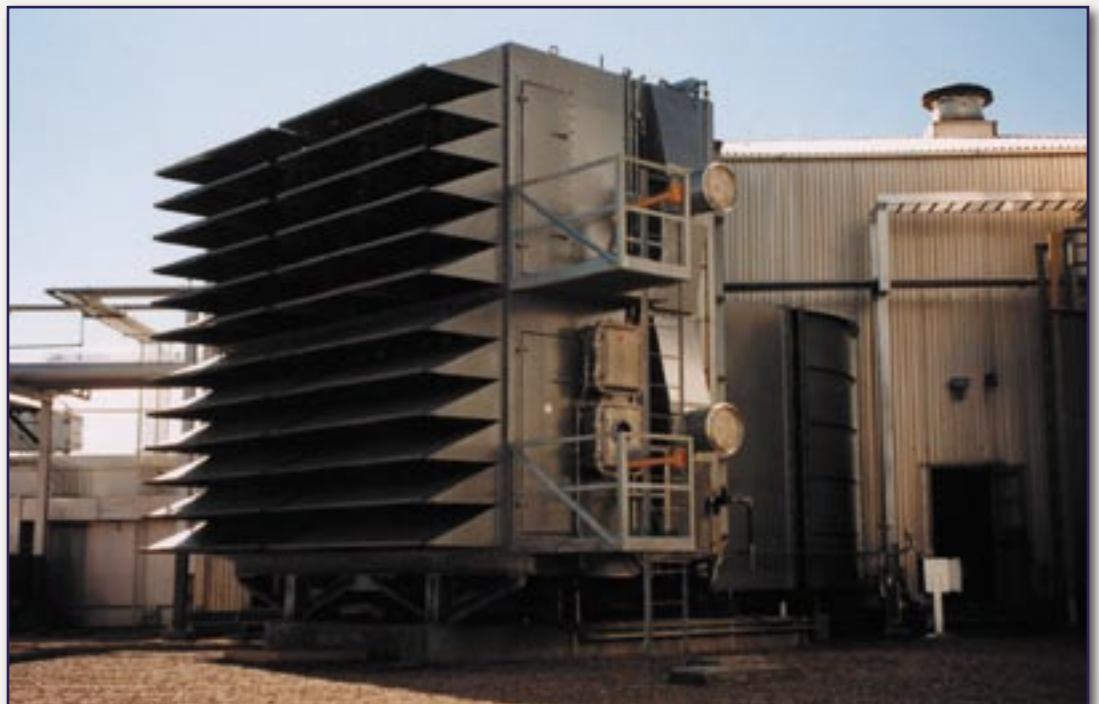
General Electric Frame 5 Self Clean Inlet Air Filter
