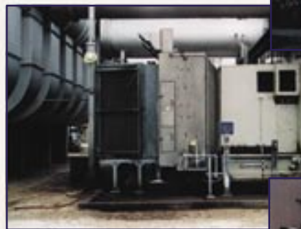
Solar Centaur retrofit evaporative cooler
