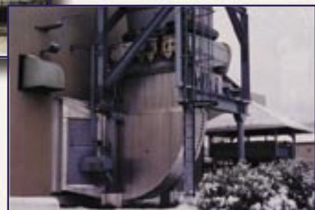
Solar Centaur retrofit oxidation catalyst
