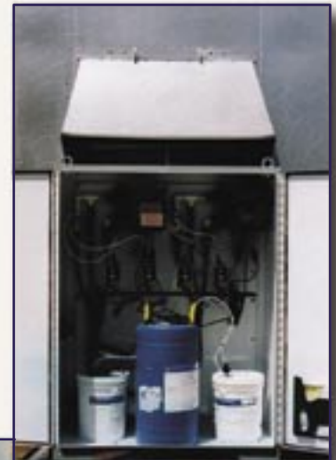
Typical chemical injection system for evaporative cooler system
