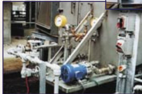
Typical recirculating pump package for evaporative cooler system
