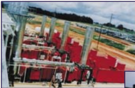
Gas turbine enclosure and enclosure exhaust cooling silencers, inlet air filters, exhaust silencer
