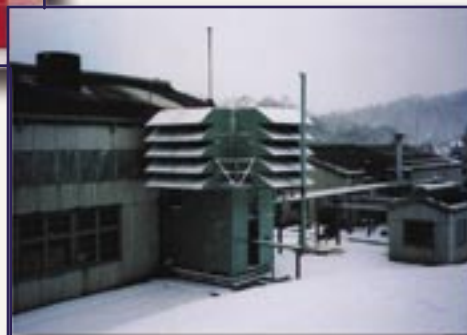
Rolls Royce Avon gas turbine compressor set inlet air filter, clean air plenum, and inlet air silencer
