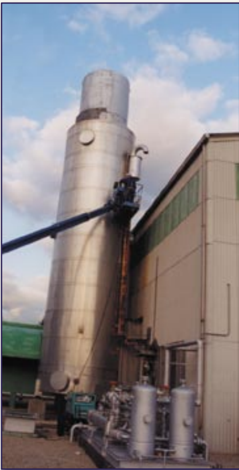
Gas Turbine Lube Oil Vent Coalescer
