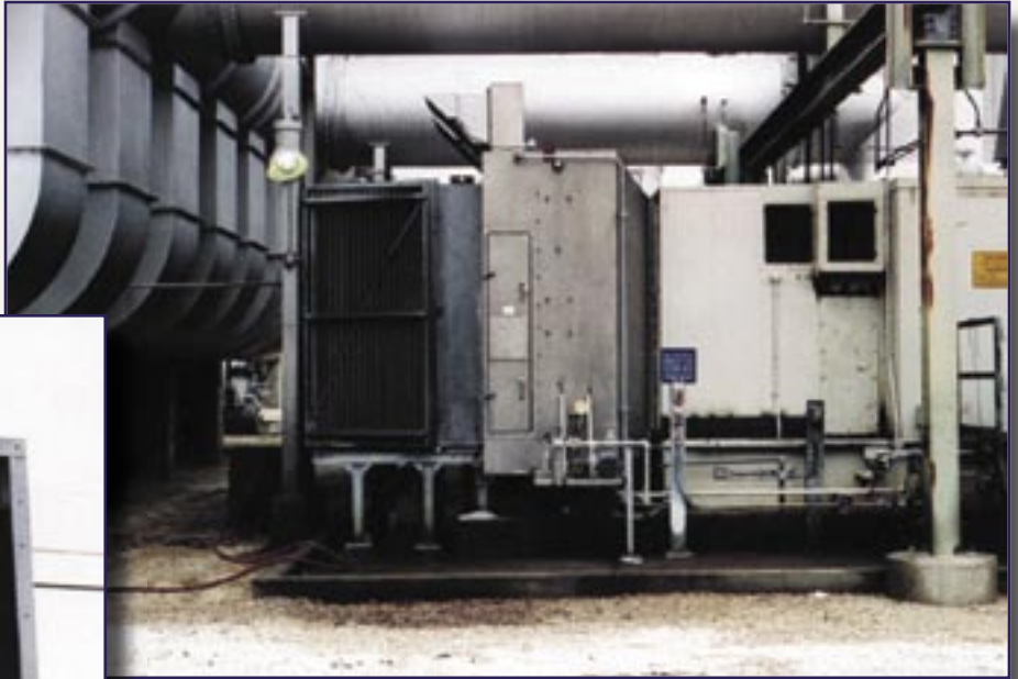
Retro-Fit Evaporative Cooler for Solar Saturn Gas Turbine
