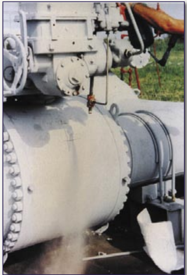
Gas Motor Operator Without Vent Mist Extractor
