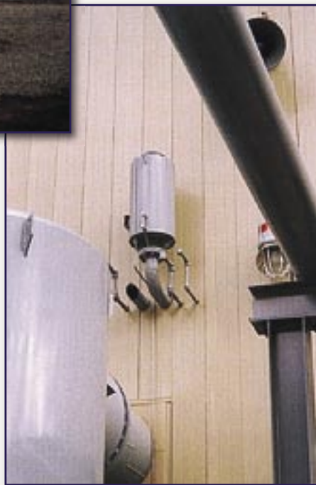
Compressor Packing Case and Dog House Vent
